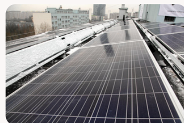
Solar panels on the roof
